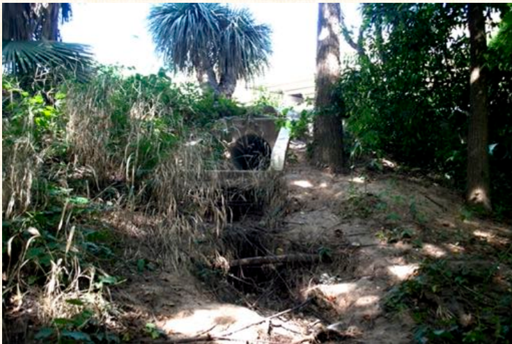
Severe rill and sheet erosion is occurring in the riparian forest downslope of the landfill parking lots. Sheet and rill erosion are severe.
